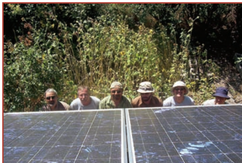
The crew of volunteer installers checks out the solar-electric awning from below.
