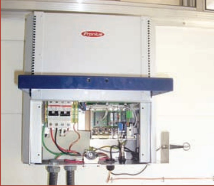
An inside look at the Fronius inverter, which converts the DC generated by the PV array into AC for house loads and the grid.
