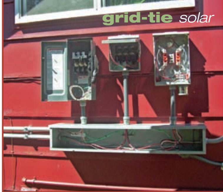
Conductors for the AC and DC disconnects, and KWH meter base with lightning arrester, are routed through a wiring gutter.
