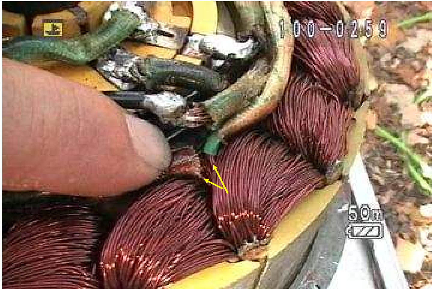
33 – Pictures of the windings...There is a low speed and high speed winding.
